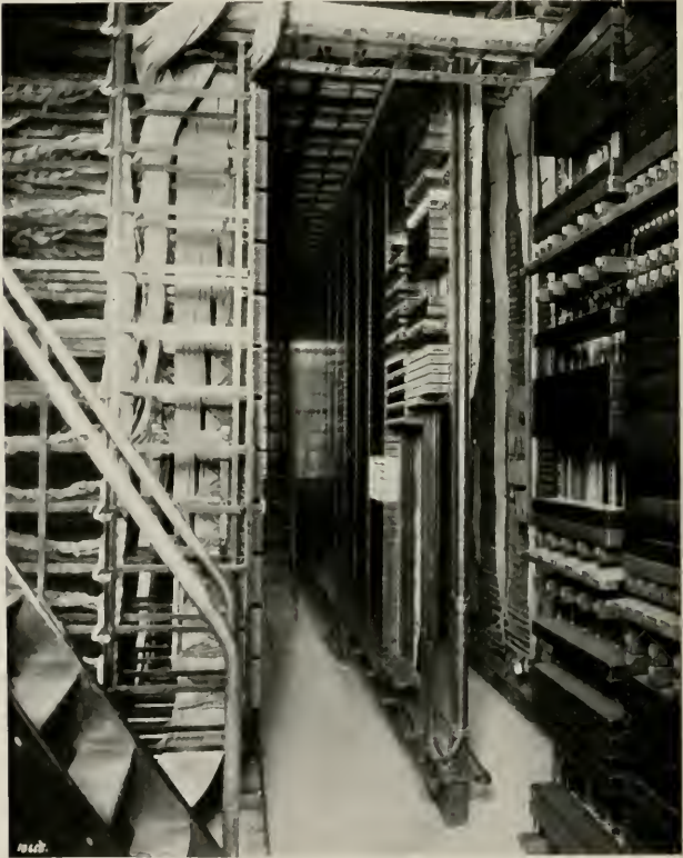
Fig. 1—Relays in a local manual office
